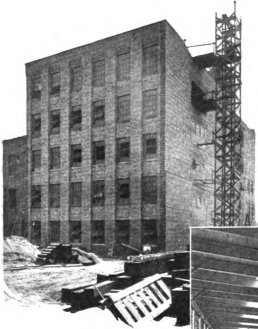
Above — Five-story addition to the factory of the Federal Rubber Mfg. Co., Cudahy, Wis. The new building will add 50,000 sq. ft. to the manufacturing facilities of the Federal company. Most of this space will be devoted to the manufacture of automobile castings
